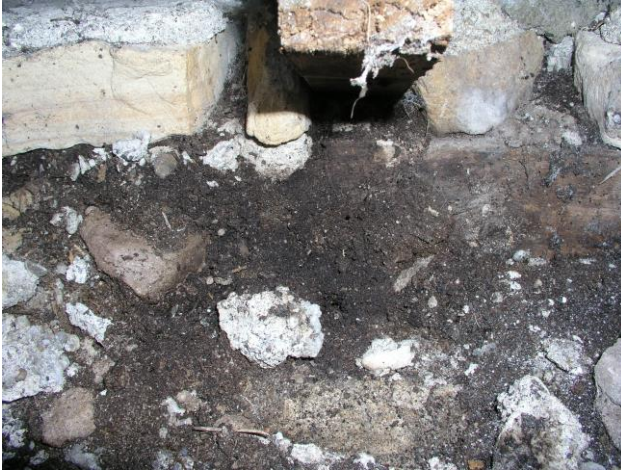
Photo showing disintegrated bat droppings beneath coping stones. If examined carefully, in the black dust exoskeletons of insects can be seen shining.
